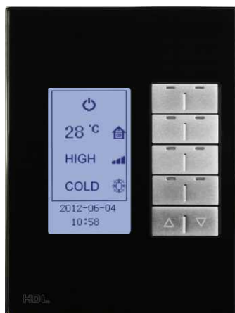
Air conditioning control interface
